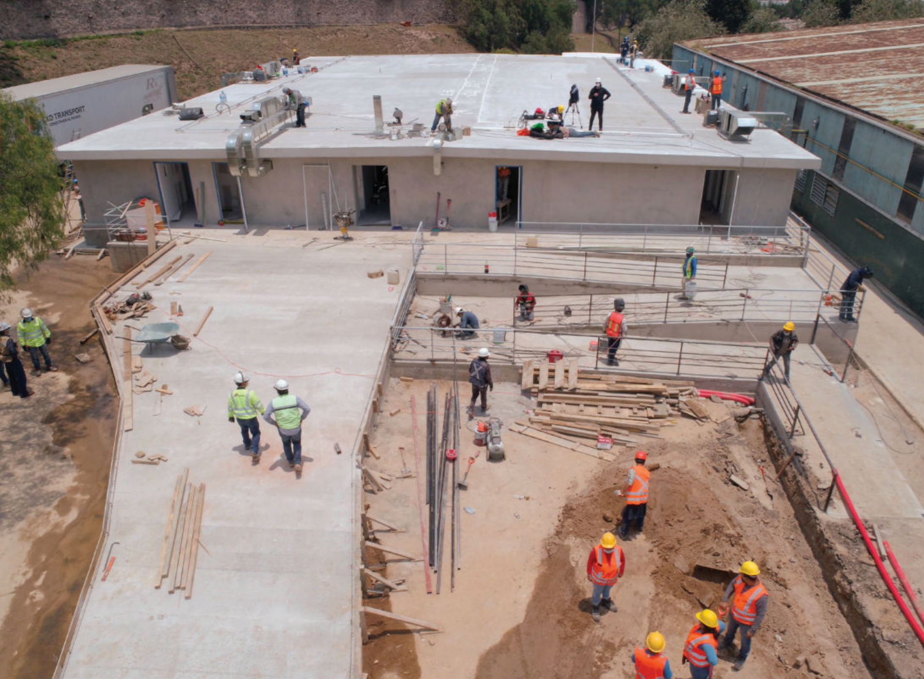
THE INSTANT HOSPITAL Cemex's prefabricated "hospital modules," designed in response to COVID-19, can be built in 15 days or less.
